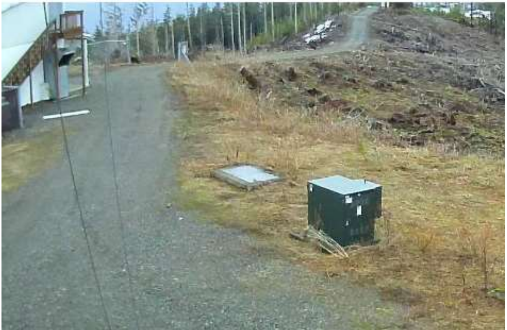
Good thing it's warming up as crews were installing safety equipment on the towers on the 24 th and 25 th .
