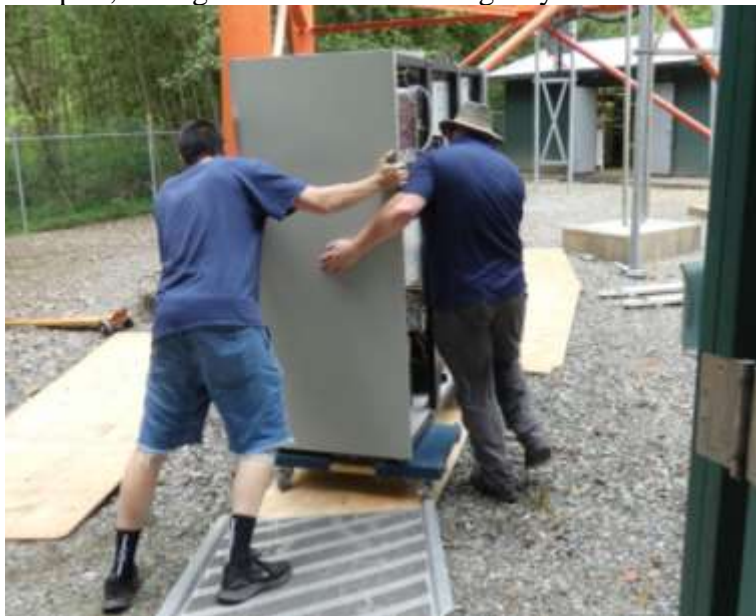
The old KNKX Transmitter heading for the building in the distance (with the open gray doors) where it will be taken apart, saving some items for emergency use.
